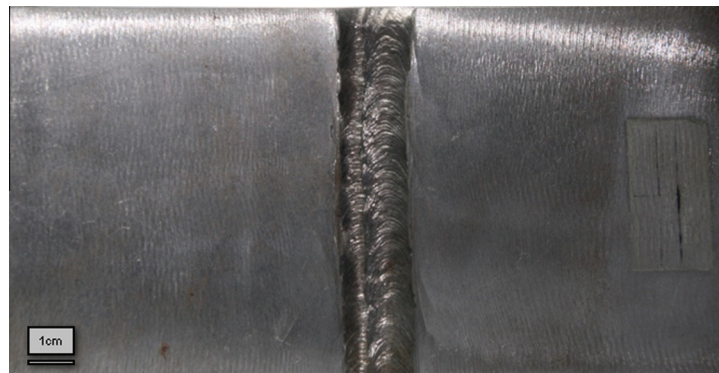
Fig. 2. Weld 1 with a toe crack.
