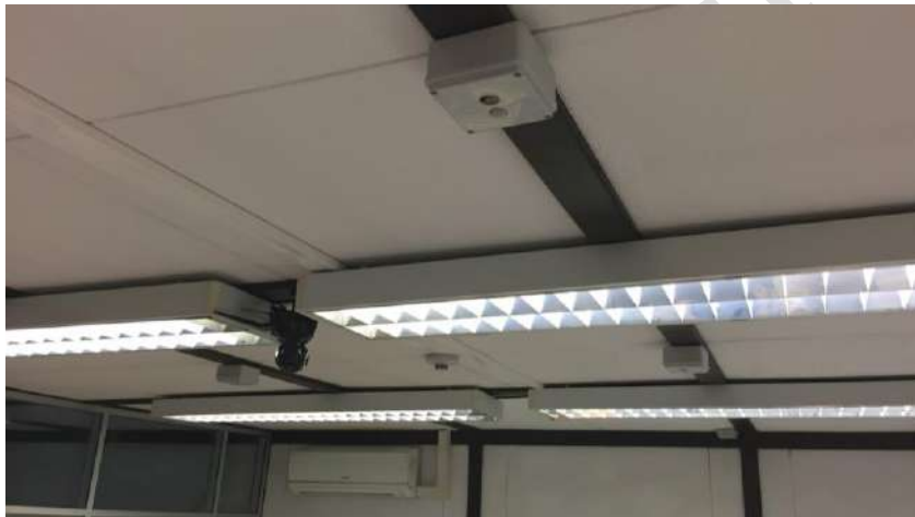
Figure 5. Sensor boxes mounted on the ceiling
