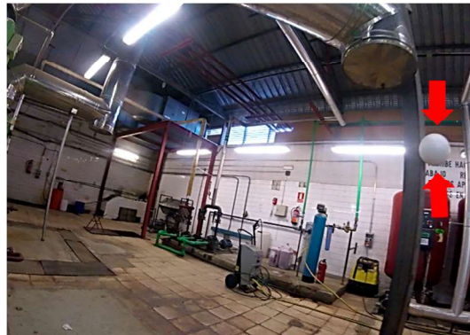
Figure 3. Sphere located in a pillar of the machine room (attached by a neodymium magnet).
