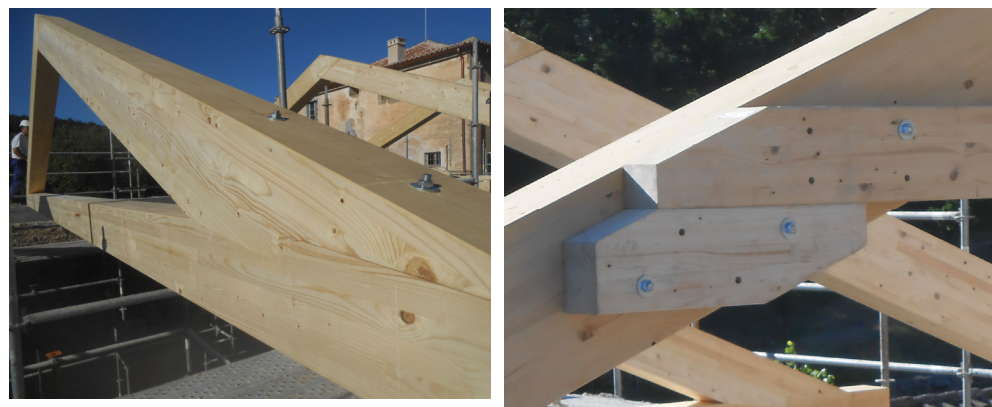
Figure A2. Examples of actual structures using dowel type joints with washer-nut endings.
