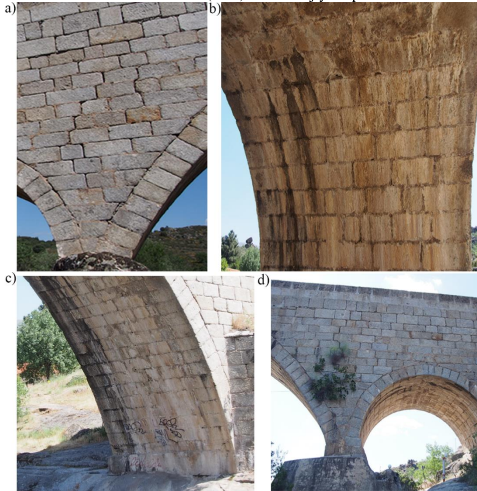
Figure 4: Current state of conservation of the bridge: a) cracks on the spandrel wall; b) Salt crusts and soiling on the smaller barrel vault; c) Salt crusts, soiling, and graffiti on the bigger barrel vault and d) higher plants on the spandrel wall.
