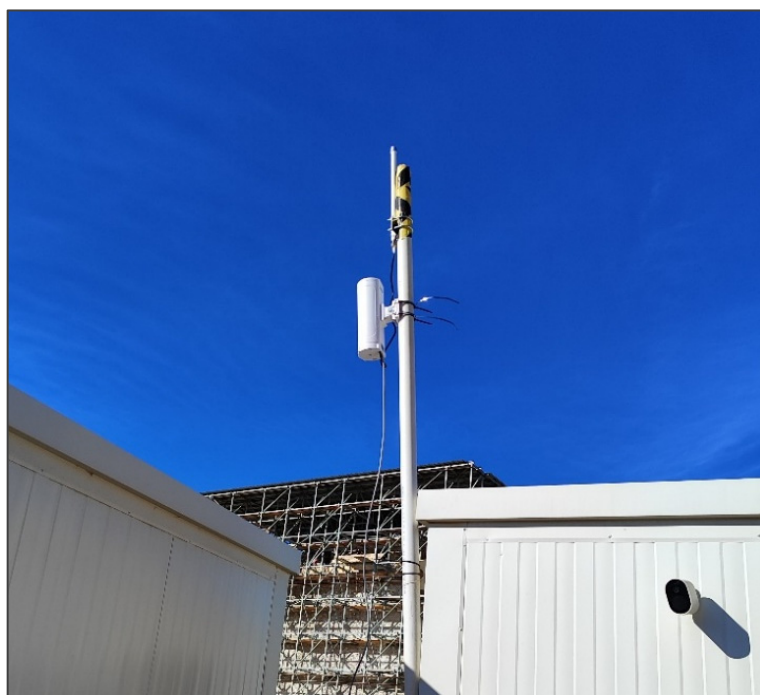
Figure 8. Placement of the Dragino DLOS8N Gateway.
