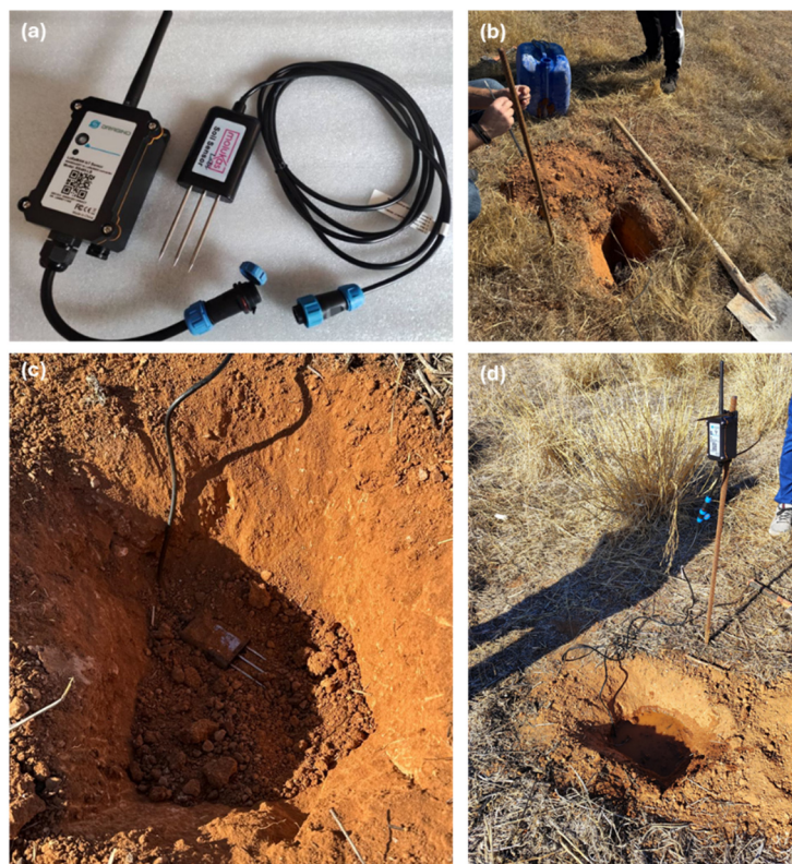
Figure 7. (a) NPK-7in1 LoRaWAN Soil NPK Sensor EU868. (b) Excavation of the hole in the soil and placement of the steel rod for the processing unit. (c) Installation of the sensor in horizontal position inside the hole. (d) Covering of the sensor with soil and controlled watering to compact the soil and ensure optimal contact with the substrate.
