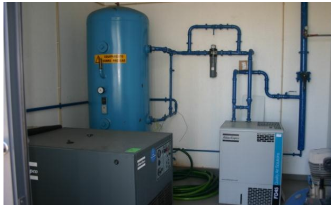
Figure 51 - Central of compressed air
