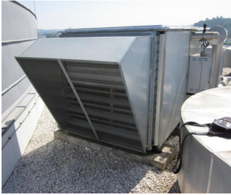
Figure 46 - AHU with new air intake
