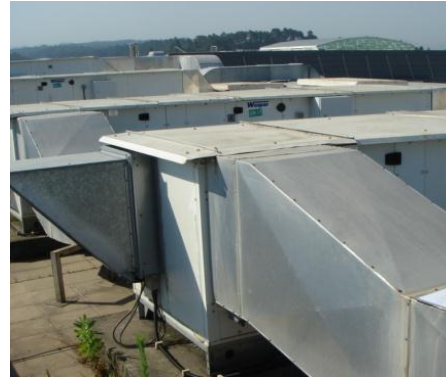
Figure 47 - AHU with new air intake and renewed air
