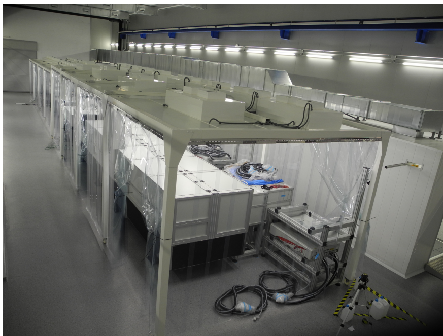
Figure 3.4: VEGA Petawatt - Picture of the on-going installation of the VEGA Petawatt laser system. This shows the optical tables with parts of the amplification stage.
