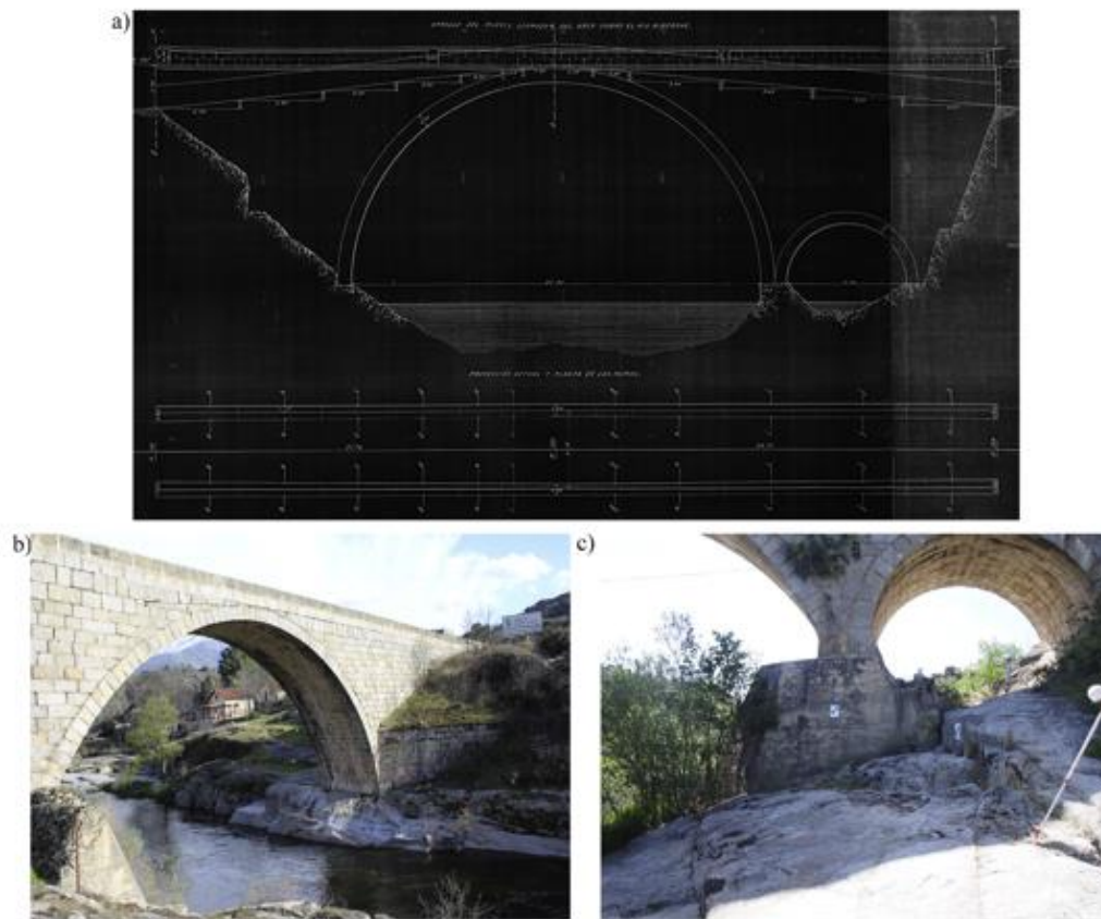
Fig. 1. The Arco Bridge: a) downstream elevation before and after restoration works; b) upstream elevation and; c) reinforced concrete layer added to the pier between vaults.
