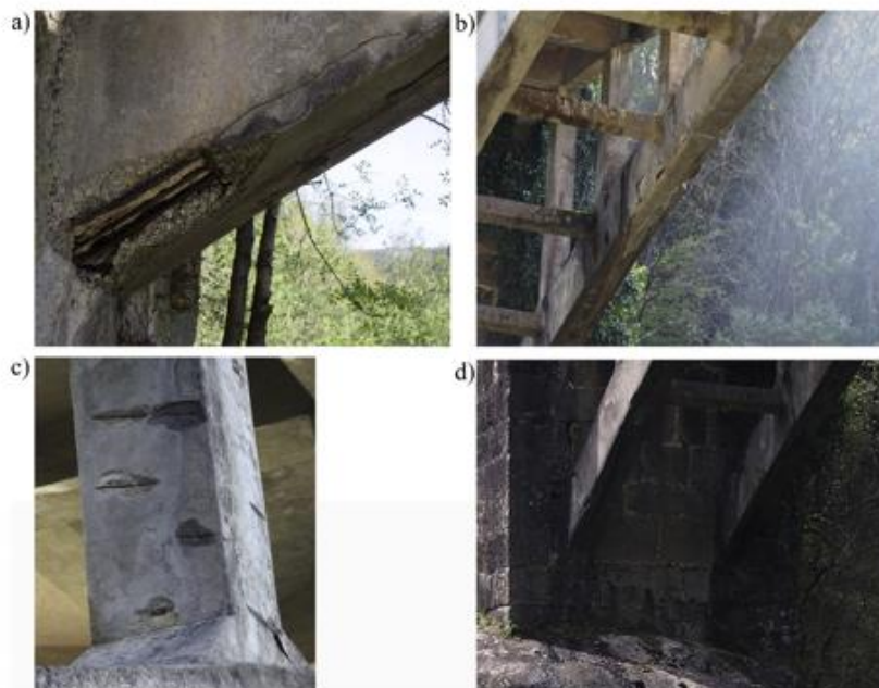
Fig. 7. Current state of conservation: a) extreme of an arch girder; b) concrete spalling on an arch girder; c) concrete spalling on a pillar; and d) cracks on the V. Minho vertical masonry wall.
