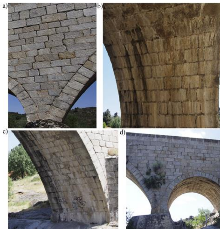
Fig. 4. Current state of conservation of the bridge: a) cracks on the spandrel wall; b) Salt crusts and soiling on the smaller barrel vault; c) Salt crusts, soiling, and graffiti on the bigger barrel vault and d) higher plants on the spandrel wall.
