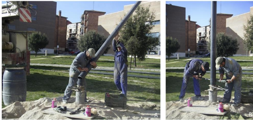
Fig. 4. Stage 2. Piped. (a) Piping the first meters. (b) Joining pipes with different tools.
