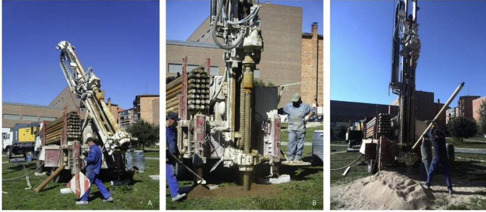
Fig. 3. Stage 1. Drilling. (a) Positioning of the drilling machine. (b) First meters drilled. (c) Adding new drilling rods.
