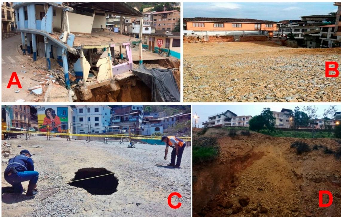
Figure 3. (A) Collapse of the Fe y Alegría School, in October 2916. (B) Technical filling done at the site in 2017. (C) Reactivation of the collapse in the place where the school was in 2017. (D) New collapse near Gonzalo Pizarro Street in 2019. Images taken from El Expreso Newspaper, Ecuador en vivo, Pichincha Universal and Arden los Socavones Facebook page.
